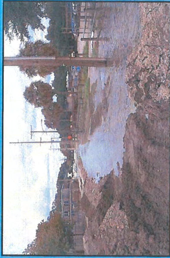
University Pump Station Force Main Break
