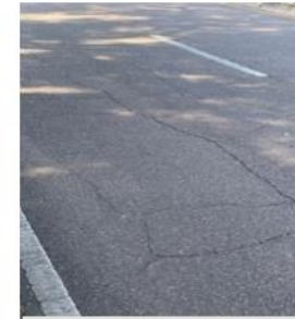
Linear / Transverse cracking
